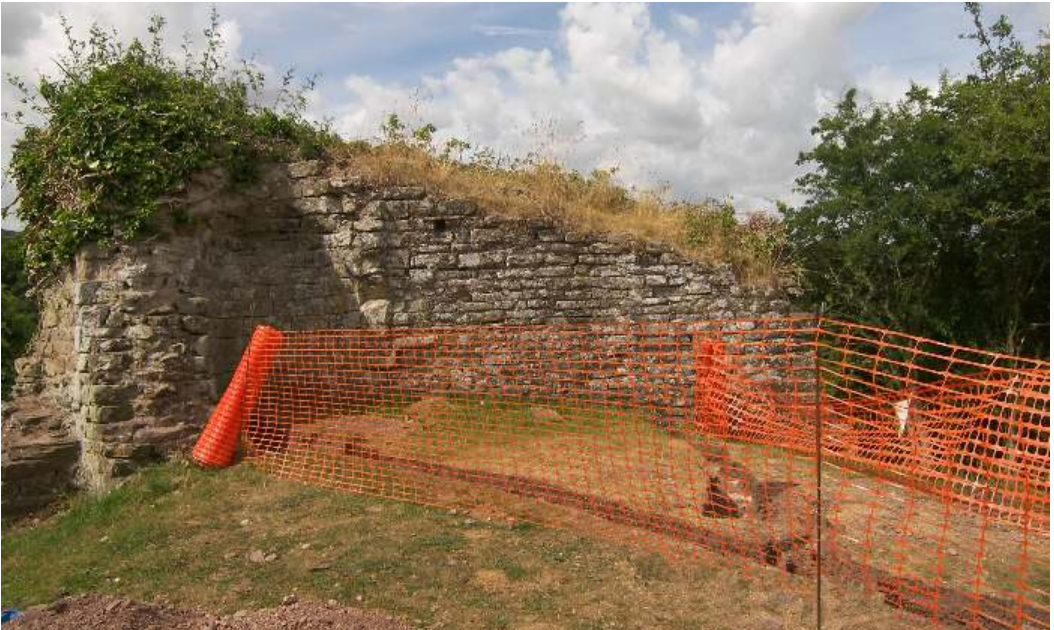
BELOW: Fig. 5. Fragment of shell wall to the south-west, (the south wall) including a pitched roof-line, a fireplace, a recess for garderobe or stair-case, a drain/urinal, part of an inward-projecting cross-wall.
