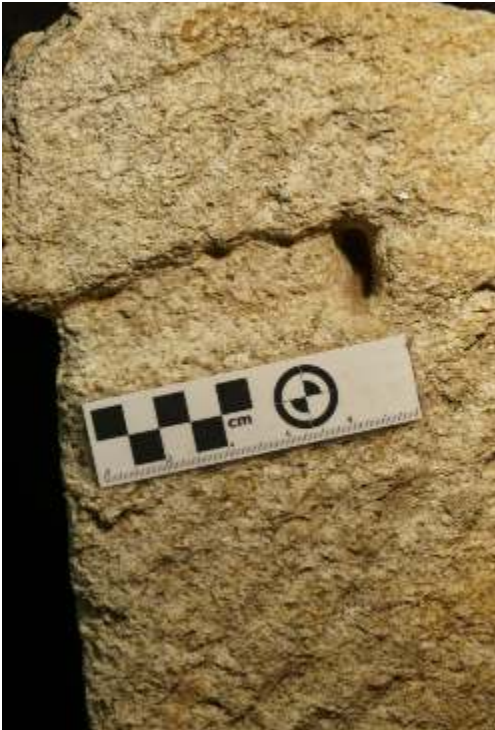
Fig. 7. Detail showing the slot for a cramp in the lowermost of the three chamfered stones, photographed in 2015.
